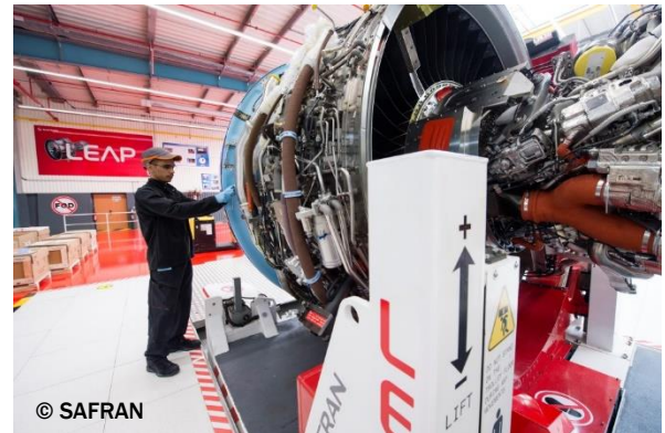
Example of complexity of existing engine installation
